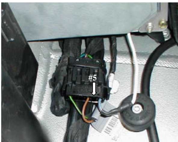
View showing Connector X9359. Cavity #5 (arrow) provides the power to Relay #2 contacts for the Aux lights. Although this picture shows a wire coming out of cavity #6, this is incorrect (don't ask). The green and brown wires are for the heated grips.
